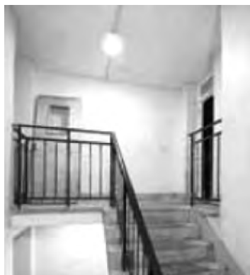
photo of stairwell with LED fitting
