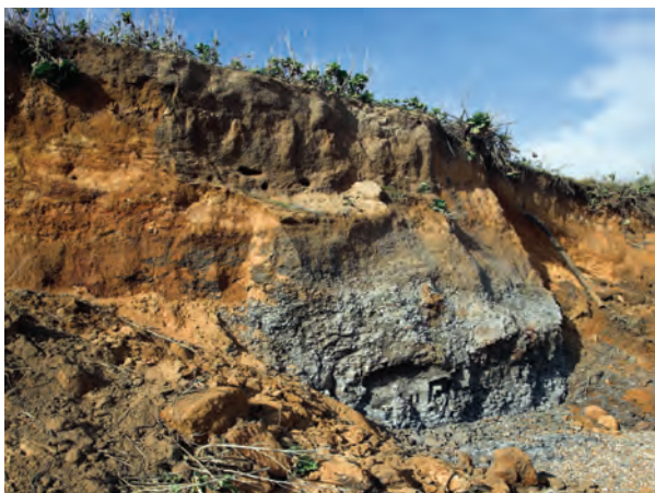
Photo 1 Cliff regrading high maintenance and high cost.
