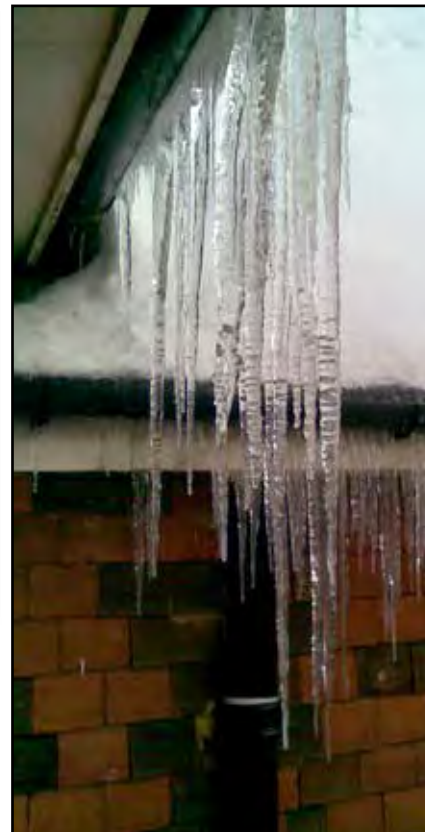
Figure 4: Icicles on guttering – a sign of long-term freeze/thaw
