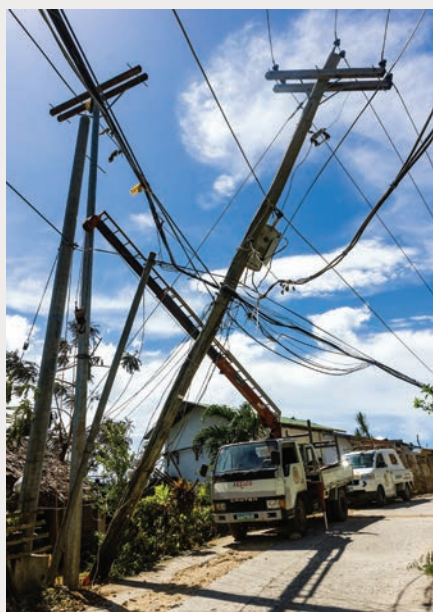
Figure 8 Damage to infrastructure Source: www.shutterstock.com; photo by Richard Whitcombe
